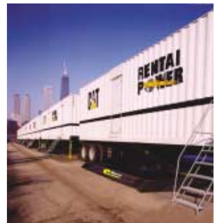
Secondary containment for generators
