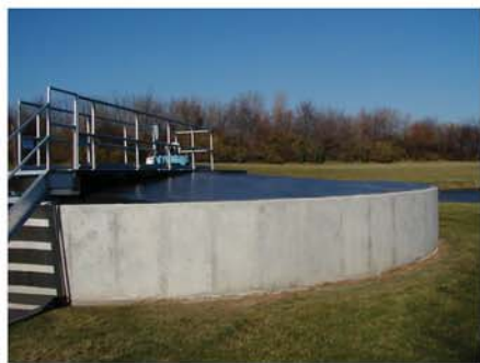
CLARIFIER COVER WITH BRIDGE
