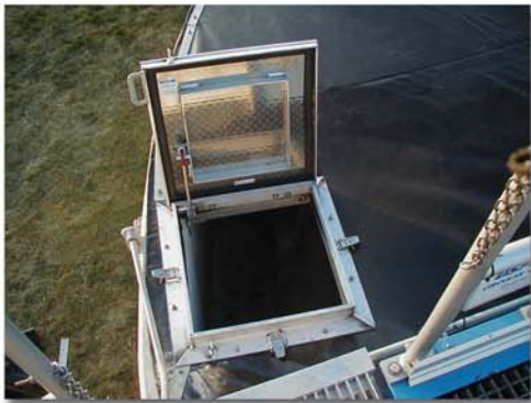
MANWAY ACCESS HATCH
